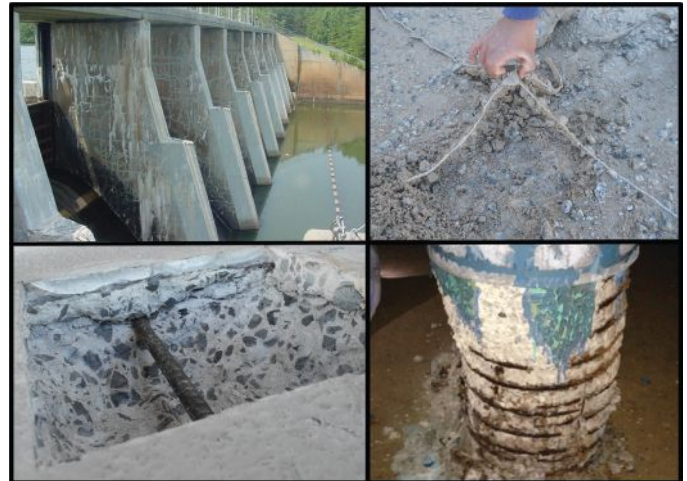
Fig. 2: Examples of materials-related distress top left to right: alkali-silica reactivity (ASR) and freezing and thawing damage (F-T); bottom left to right: corrosion, and chemical attack / corrosion
